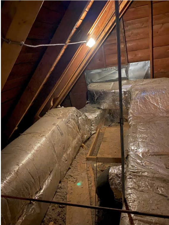
Photo 18: Notched Rafter in the Attic (Low Roof)
