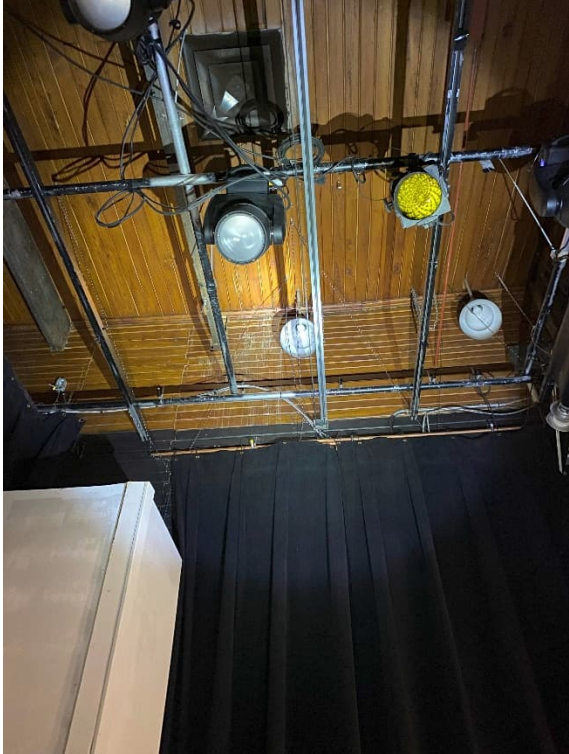
Photo 1: Water Stains near the Junction of Lower Roof and Main Roof
