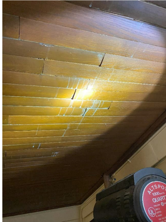
Photo 3: Water Stains near the First Window from the Northeast Corner
