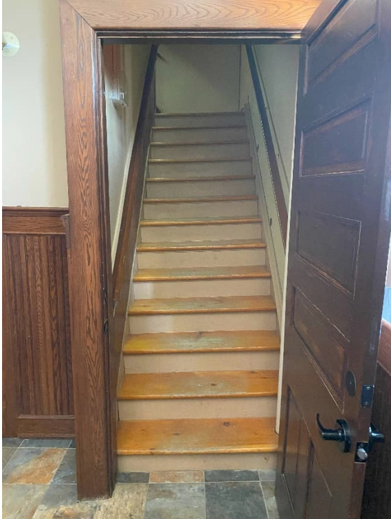
Photo 21: Unlevel Stairs at the Northeast Corner of the Building
