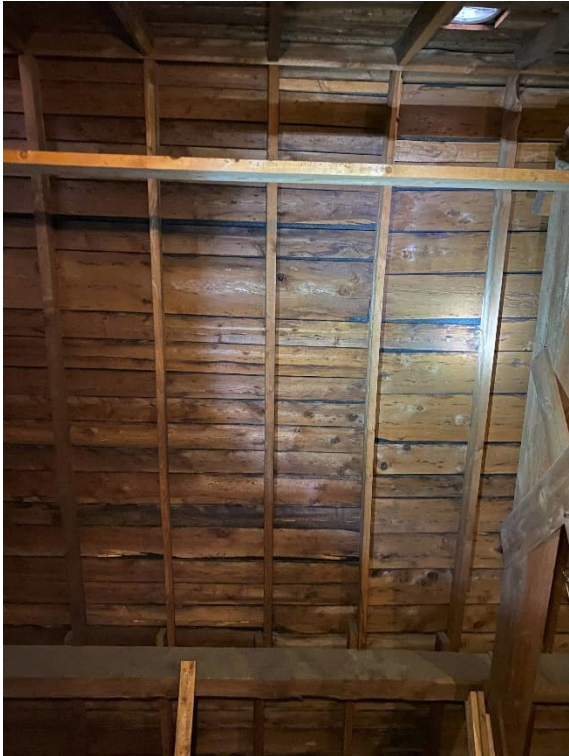
Photo 15: Gaps between the Wooden Planks at Main Roof
