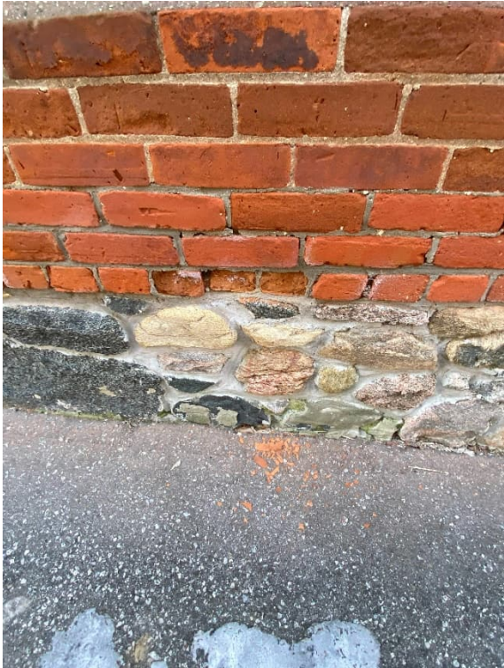
Photo 24: Brick Spalling on North Exterior Wall
