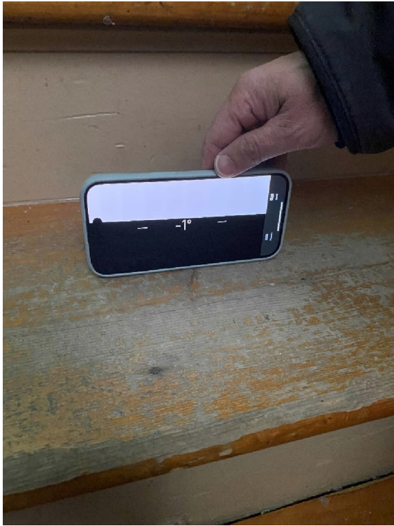
Photo 22: Slope Measurement of the Unlevel Stairs
