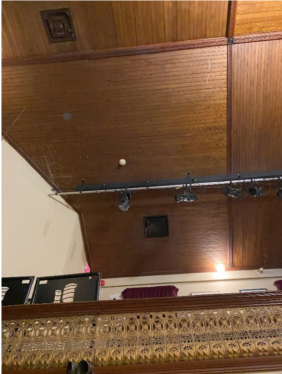
Photo 2: Water Stains beneath the North Chimney
