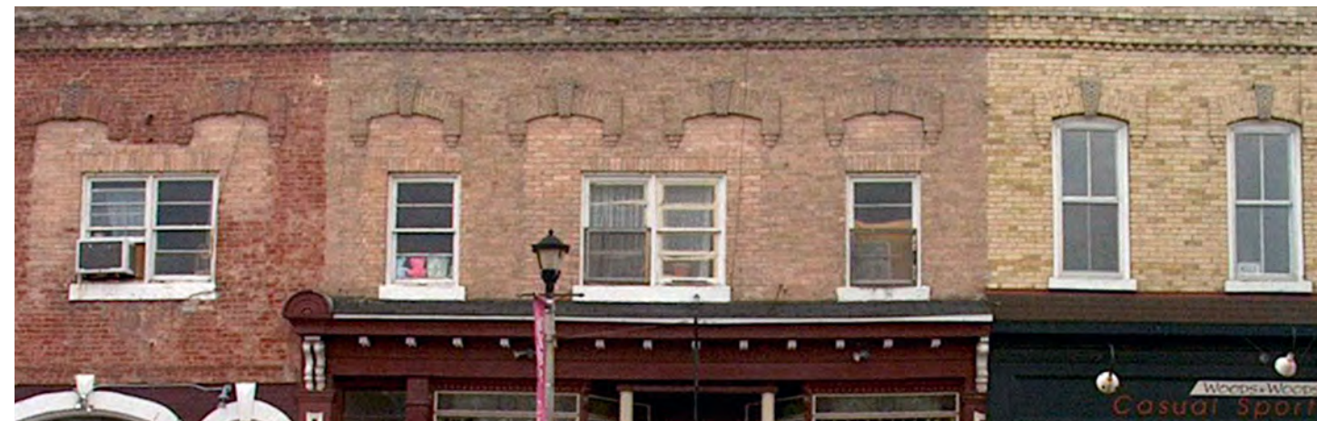
Figure 19 In situations where the original windows have been removed and window openings filled in, consult a restoration architect or a heritage contractor prior to breaking open the masonry mass.
